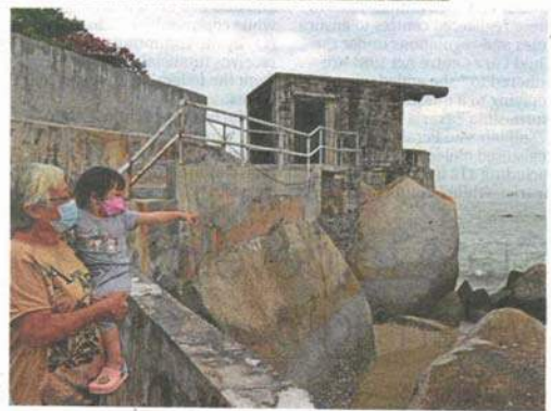
The Tanjung Tokong pillbox is also in bad shape.
